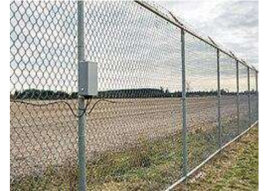
Perimeter intrusion detection
